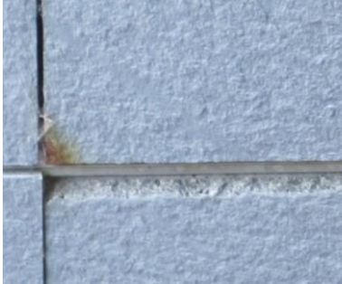
Figure 15. Spalling of the panel.
