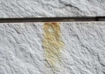
Figure 16. Red runoff stain.
