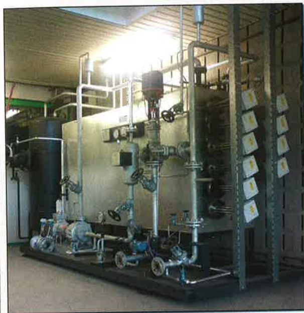
Heat source: Thermal oil boiler 250kW, Maxxtec
